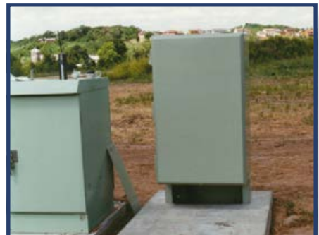
TELECOMMUNICATION CABINET BASE
