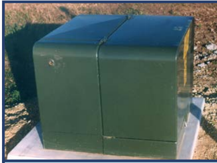
SINGLE PHASE TRANSFORMER BASE
