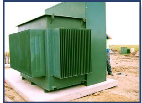
THREE PHASE TRANSFORMER BASE
